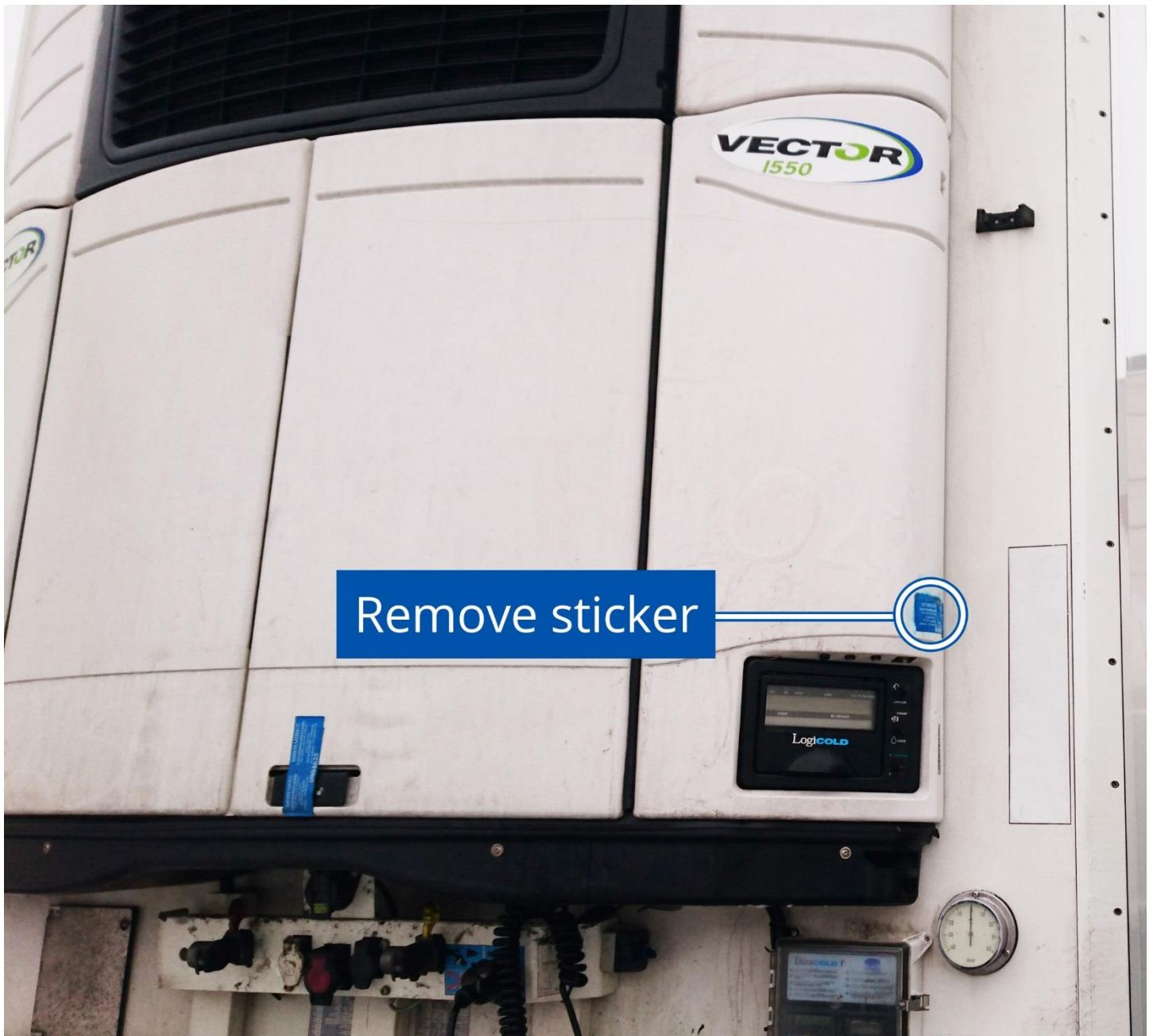
Figure 2 Fuse panel stickers location
